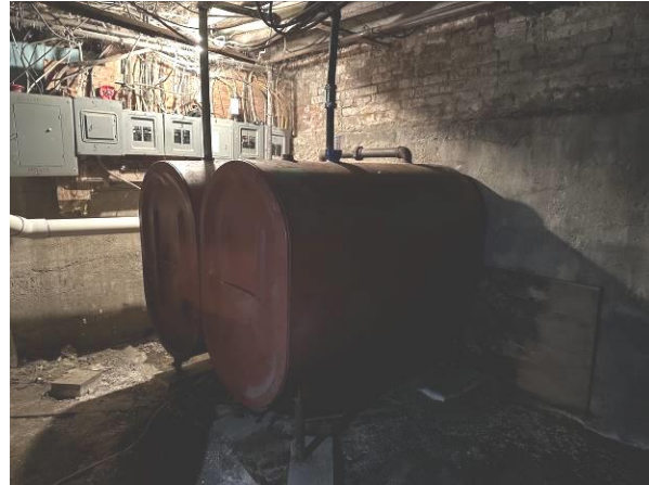
Photo No. 2 Fuel oil ASTs located on the southwestern portion of the basement of 2 State Street.
