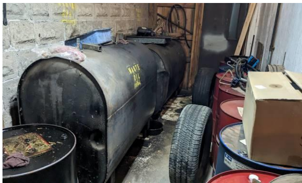
Photo No. 11 Two (2) used oil ASTs stored along the northern wall of the southern storage area.
