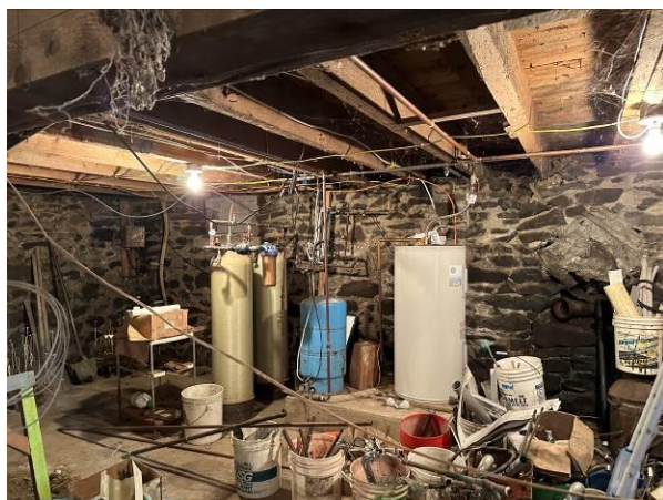
Photo No. 5 16 Charles Street water filtration system located in the basement.
