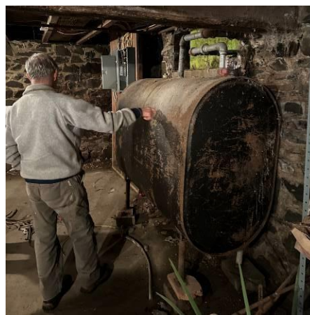
Photo No. 6 16 Charles Street fuel oil AST located in the basement.
