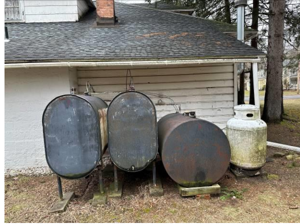
Photo No. 14 50 State Street heating oil ASTs adjacent to the east of the residence.
