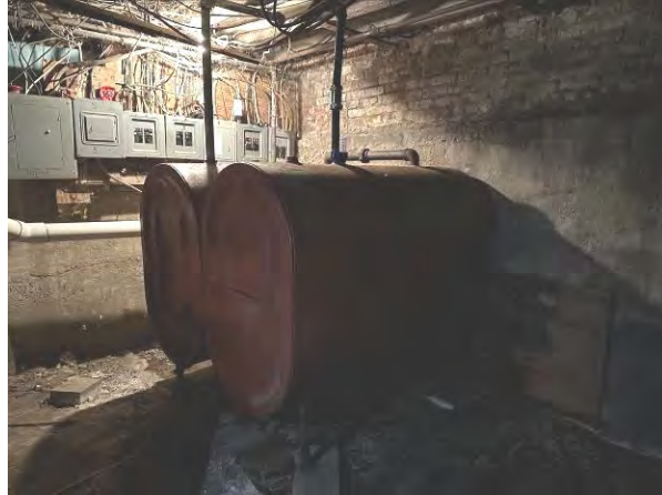
Photo No. 2 Fuel oil ASTs located on the southwestern portion of the basement of 2 State Street.
