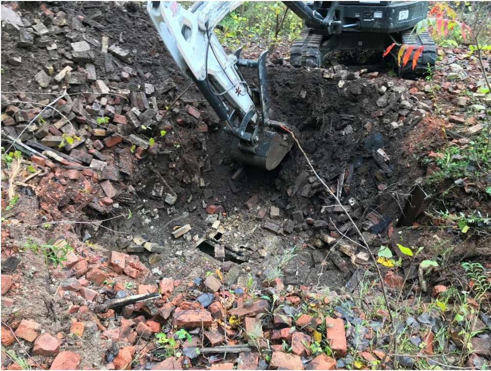
1.) Test Pit 1: Excavation to concrete slab. Excavator was able to punch through to chamber below.
