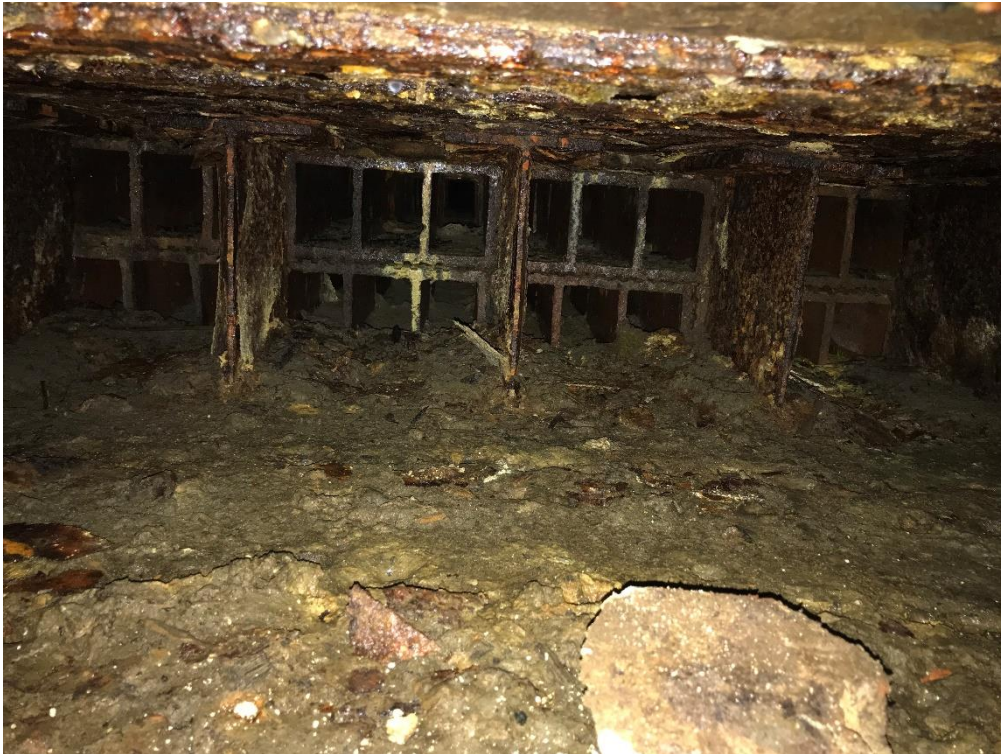
2.) Test Pit 1: Looking South away from river. Depth of chamber approx. 1 foot.
